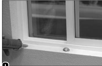
8 On the sill area, apply 1-inch balls of polyurethane construction adhesive three inches from each end and six inches apart.
