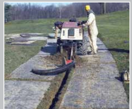
Trenching becomes much easier when AlturnaMATS® "roadway" straddles the trench. There's no damage to fairways.
