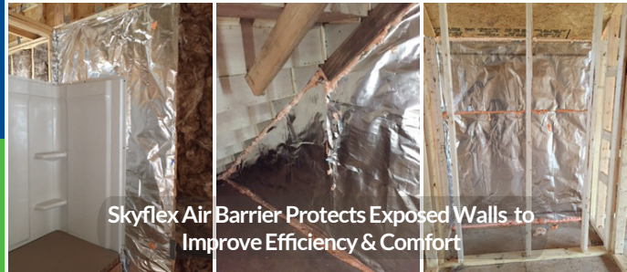
Wall Exposed to Attic with No Protection
